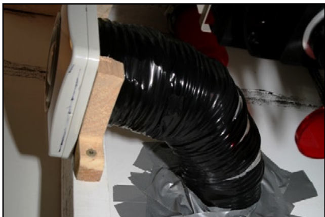
Fan ducting for air-out removal of fumes and chemical smells.
