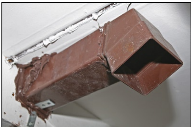
Ceiling air-in ventilation to allow for fresh air into the darkroom.
